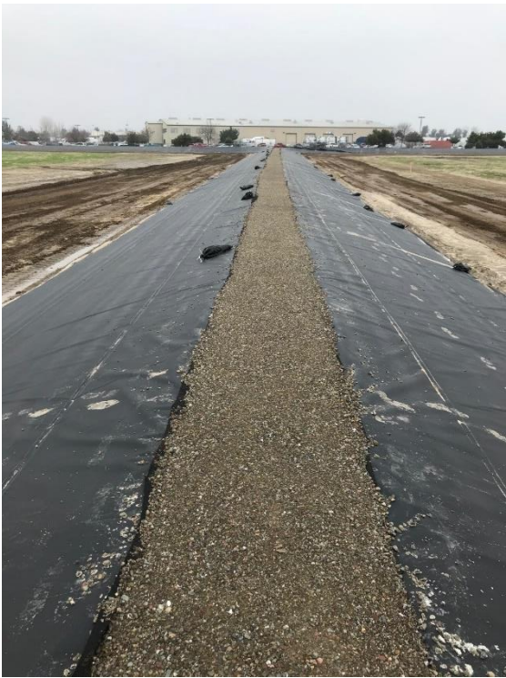
Photograph 4 - Example of Percolation Basins in Lathrop, CA with Side Wall Liner System, Modern Percolation Basins are Shallow for Frequent Cleaning and Restoration of Capacity
